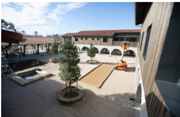
This is the central square of the Village Landais, the Bastide. It will host the following: health centre, auditorium, sport's room, activities' room, hairdresser shop, small marketplace, multimedia library, restaurant.
