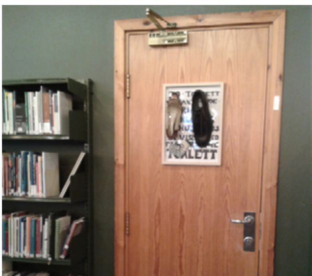
Another toilet before the adaptation.
